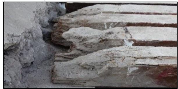
Figure 3. Deterioration in the ends of the beams
